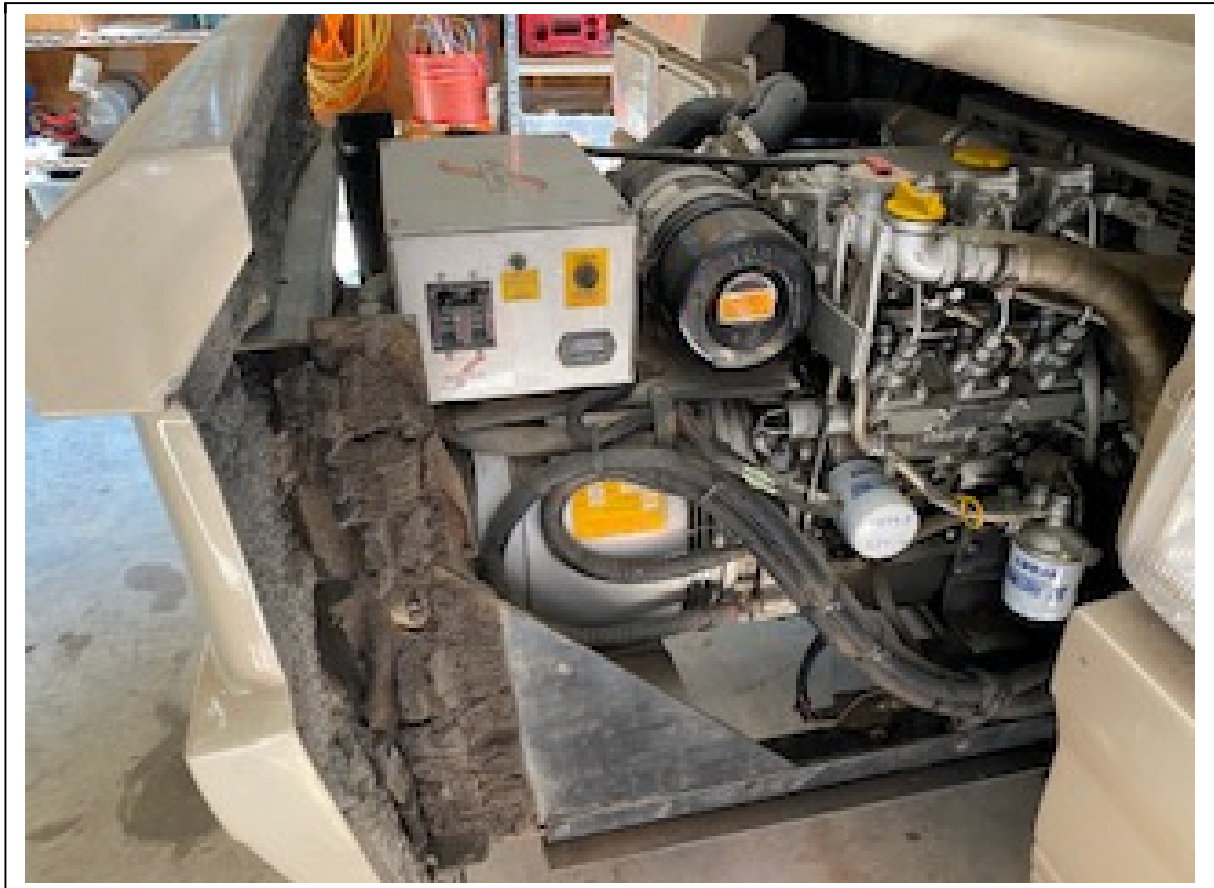
Photo # 6 Description: Powertech generator
