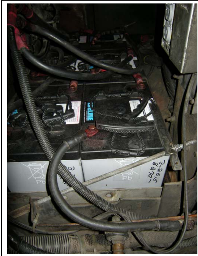
Photo # 14 Description: New Lifeline AGM batteries
