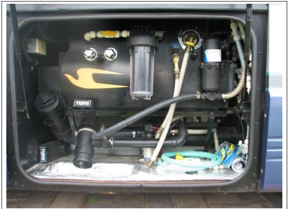
Photo # 12 Description: Water/utility bay
