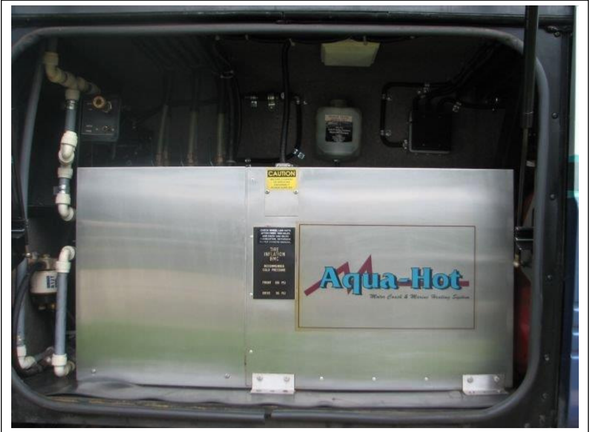
Photo # 13 Description: Modern Aqua-Hot hydronic heating system
